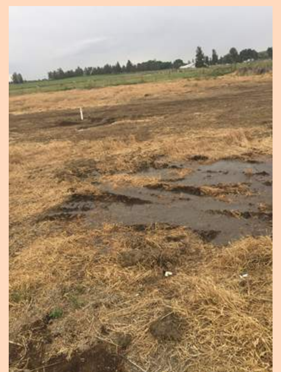
Photo 4. Surfacing effluent in drainfield
