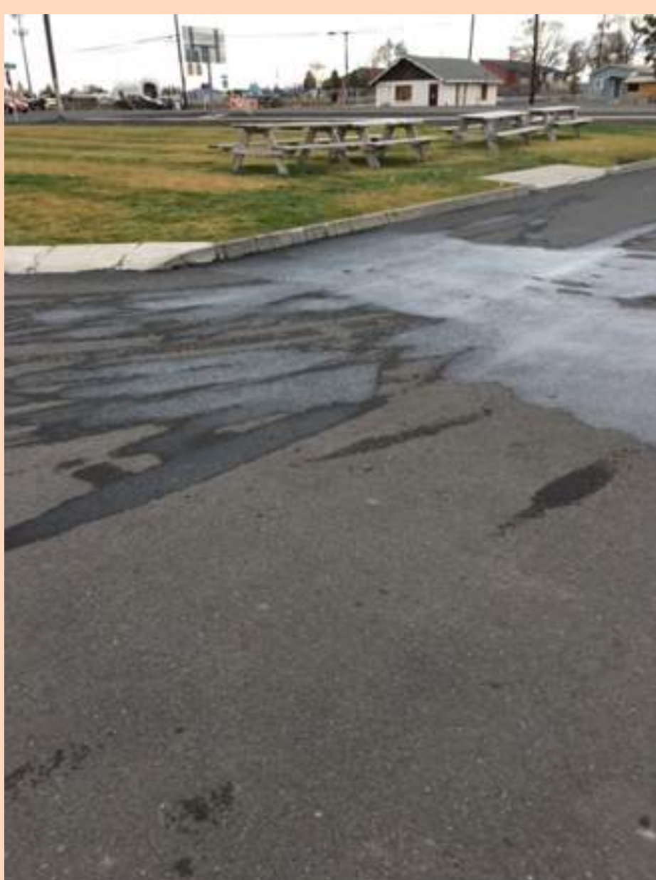
Photo 1. Sewage overflow in public parking lot
